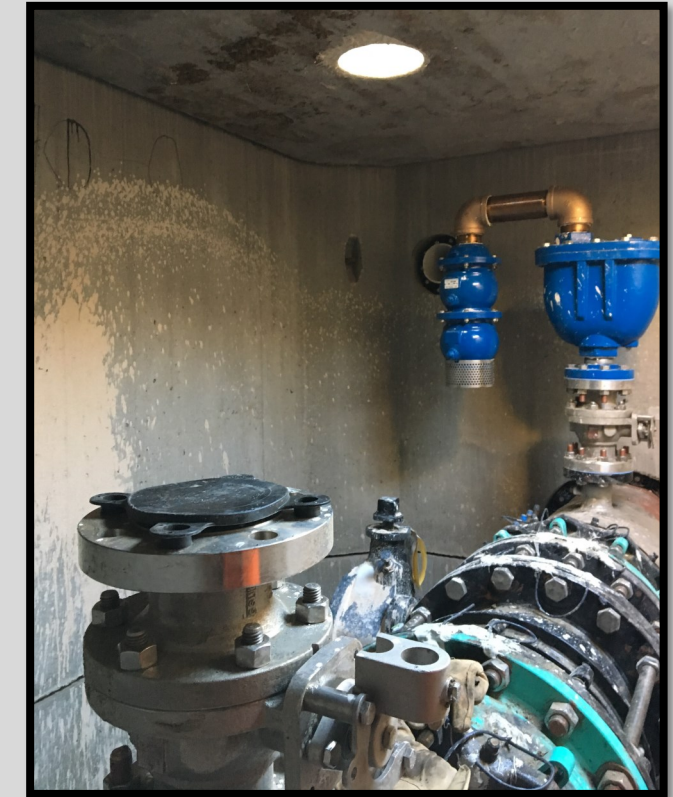
Inside the air release and valve combination vault.
