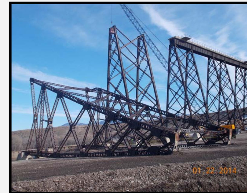
One of Two Towers Tipped Over.
