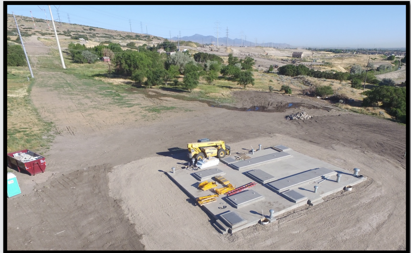
Aerial view of the Jordan Narrows Pipeline Interconnection vault.
