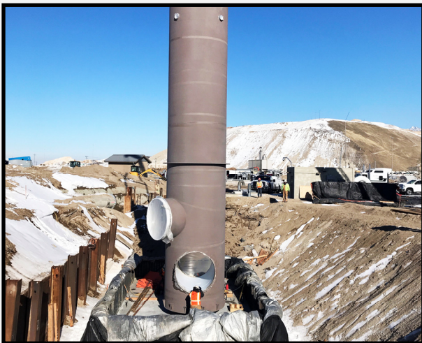
Point of the Mountain stand pipe.
