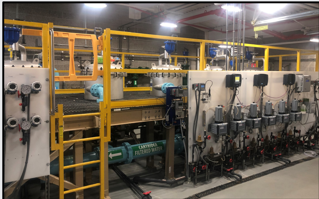
Inside the process room with 5 filters and the chlorine metering system.
