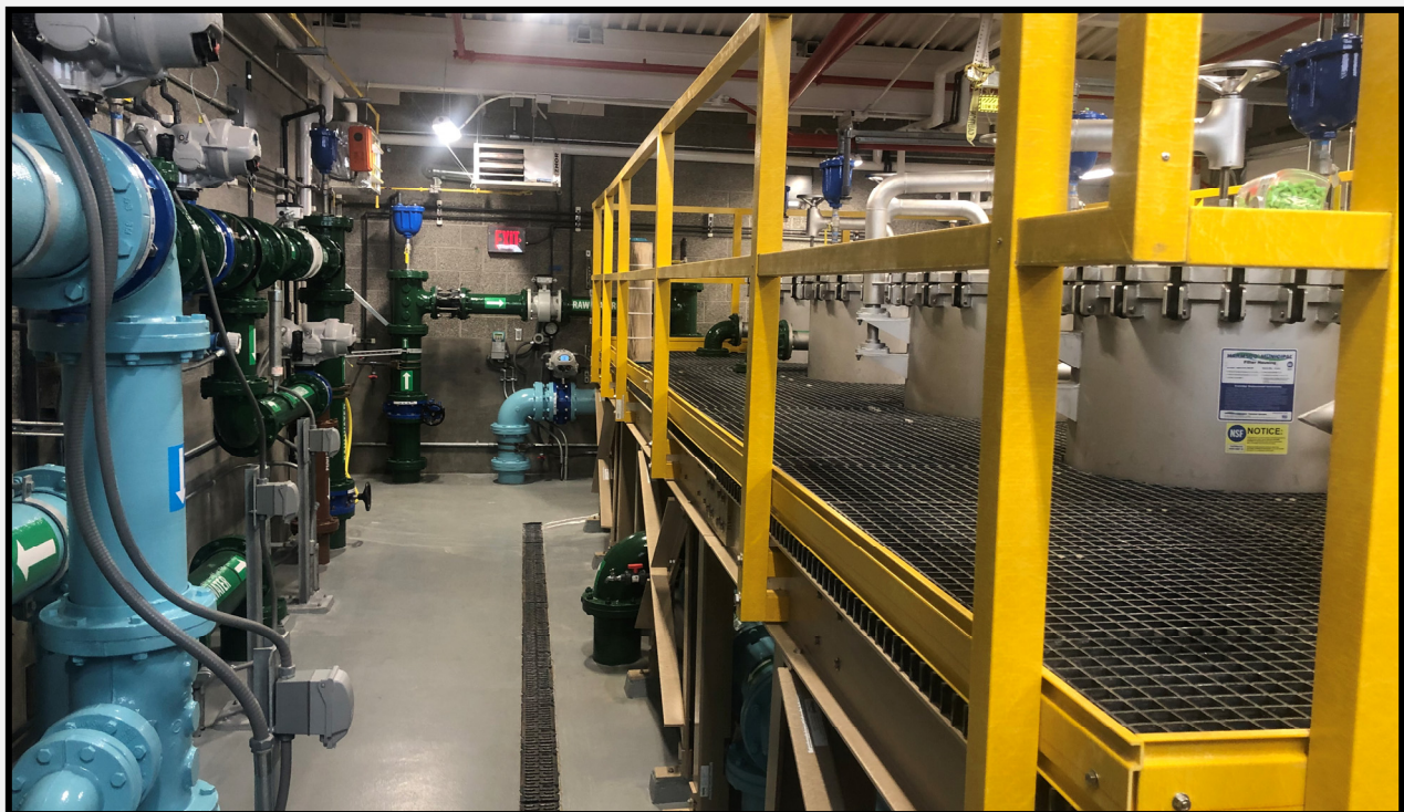
Inside the process room of the 2 wells entering the plant and the 5 cartridge filters with fiber grating access.
