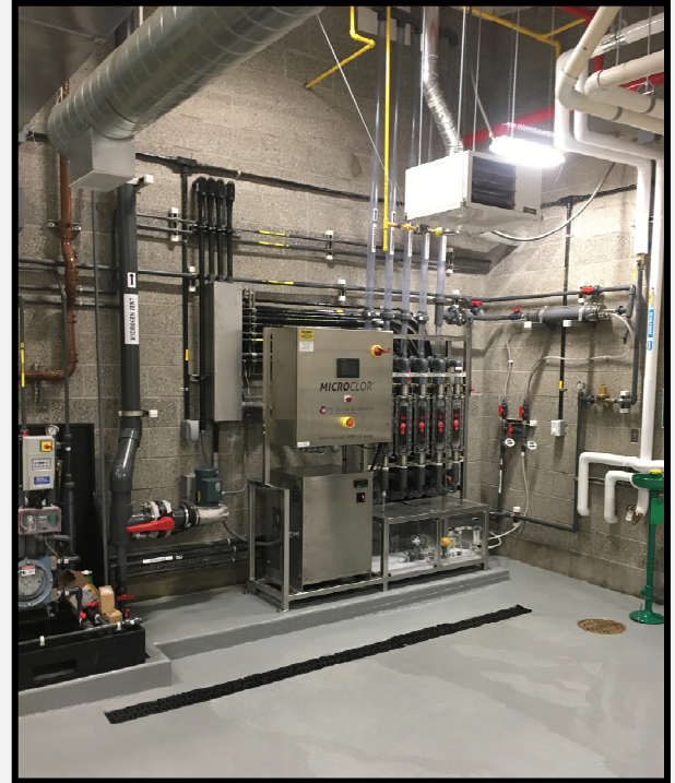
The sodium hypochlorite system inside the chemical room.
