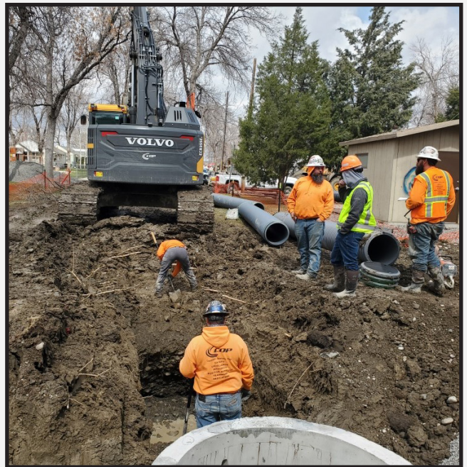
18" Storm Drain installation at Russel Park, just northeast of the new storm drain detention pond.
