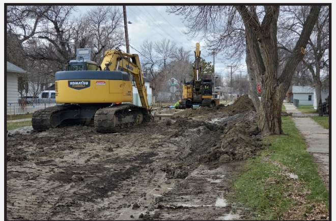
Water mainline installation on South 4th Street. The existing soil conditions have been a challenge following rain/snow events.
