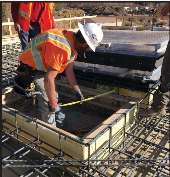
Completing the final touches in prep for casting the pump station lid.
