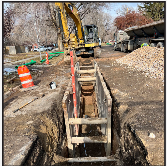
Subcontractor Gallegos Construction shored to install a new 8" sewer main on Polk Avenue.
