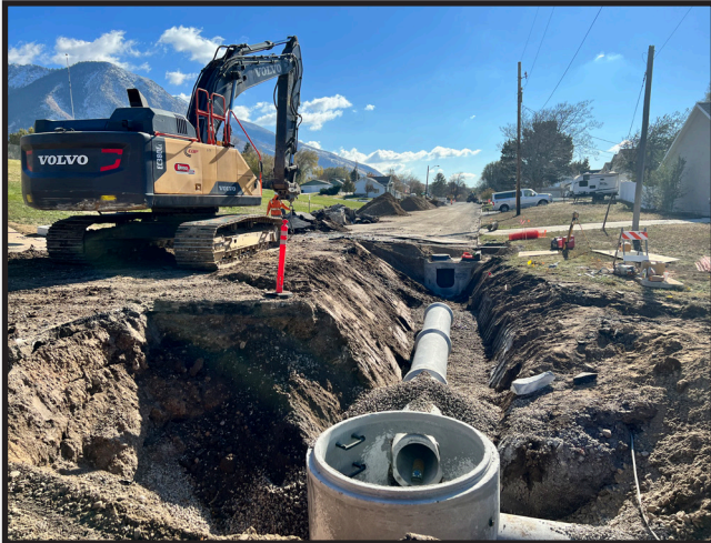
COP Crew installed new Storm Drain Manhole with 24" RCP Storm Drain Main
