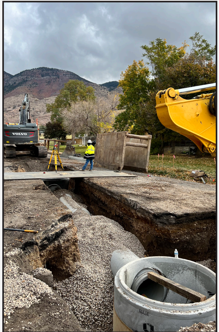
COP Crew checking the grade and verification of design flow line elevation on the new Storm Drain Manhole and 30" RCP Storm Drain Main.
