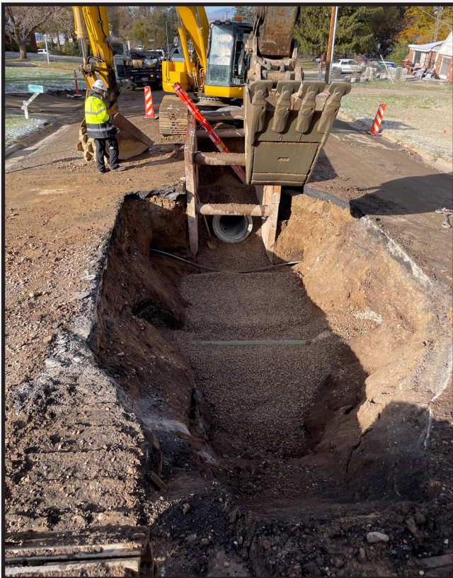
COP Crew lowered an existing sewer lateral that conflicted with the design grade of the 24" RCP Storm Drain Main.
