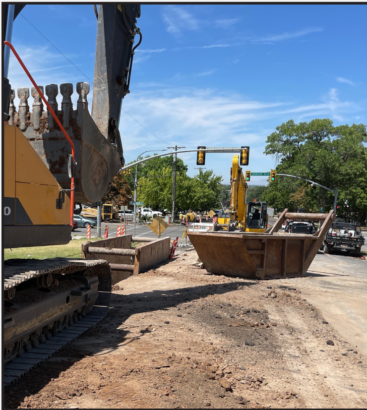
COP Crew began construction of the 30" RCP Storm Drain Main at 22nd Avenue & Harrison Boulevard.
