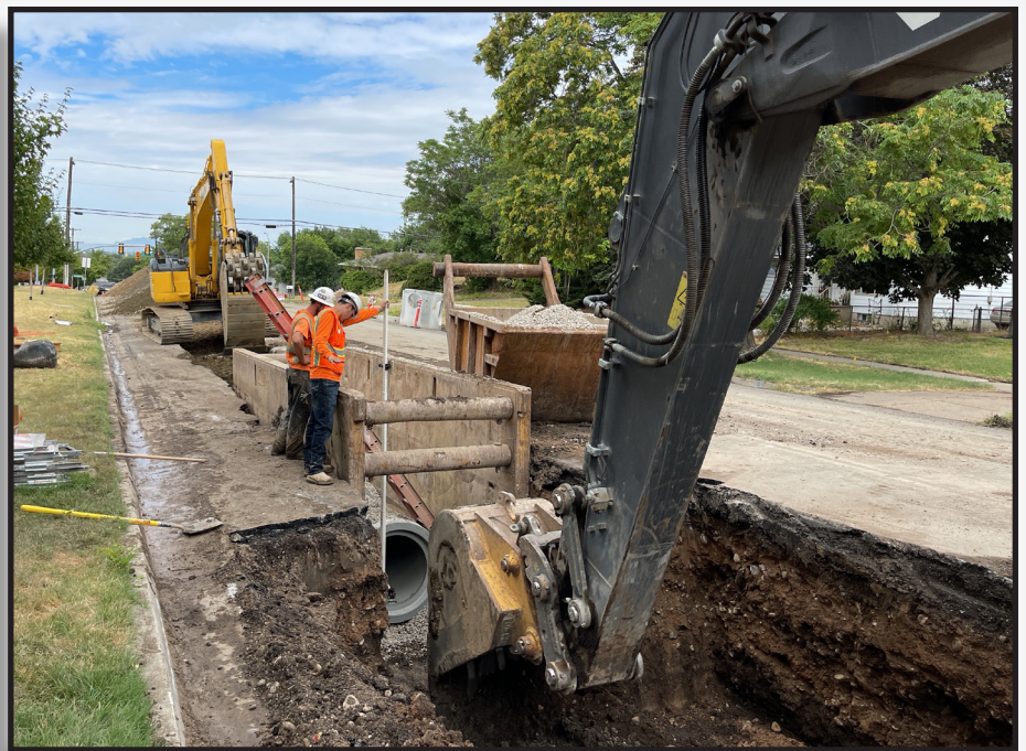
COP Crew checking grade and verification of design flow line elevation on the 30" RCP Storm Drain Main.
