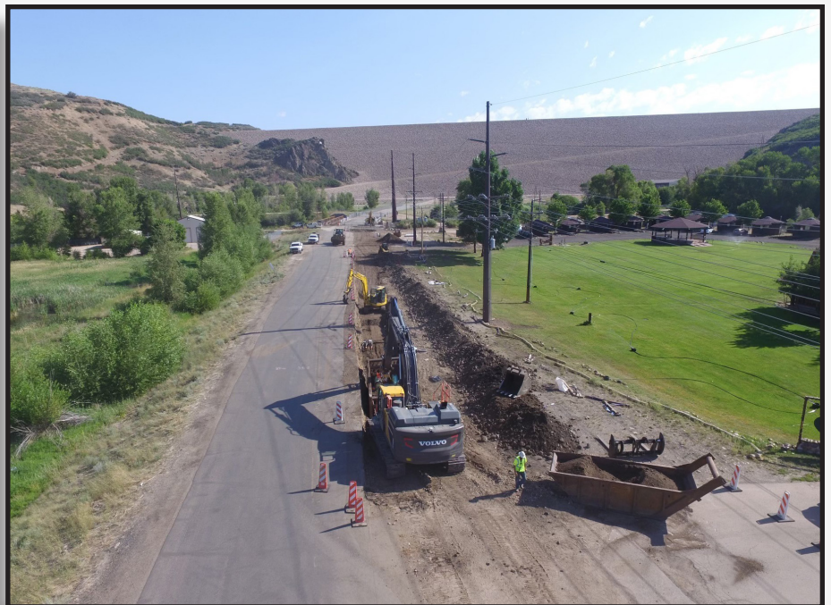
Overview of the crew backfilling the trench zone on the north end of the project.
