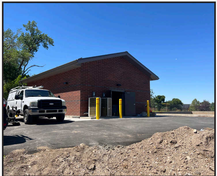
Pump station building brick exterior done by Rocky Mountain Masonry. Metal roofing, soffit, fascia, gutter and downspouts installed by Omega Metals
