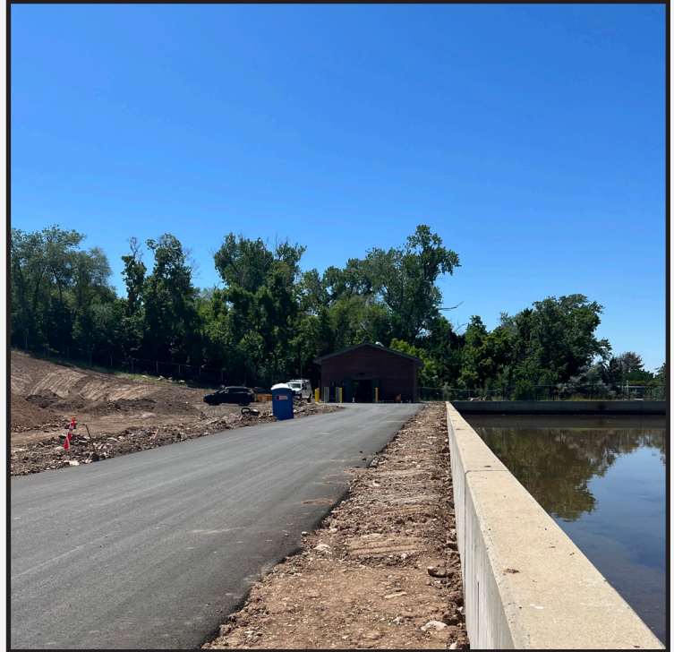
Newly paved access road to Weber South Pump Station installed by Ridge Rock.
