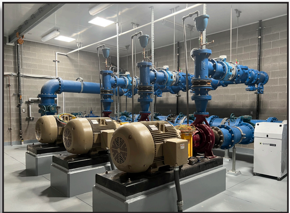
125 HP Horizontal Centrifugal Booster Pumps- coupled to suction and discharge piping.
