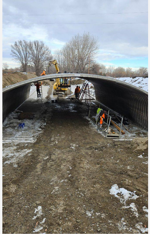
Tightening the bolts and installing the ribs adding strength to the structure
