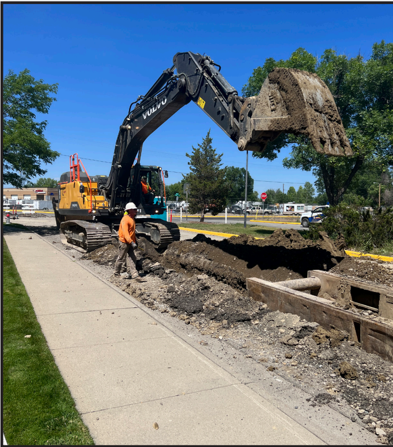
12" Water Main Replacement near the intersection of Parkway Lane & King Avenue East.
