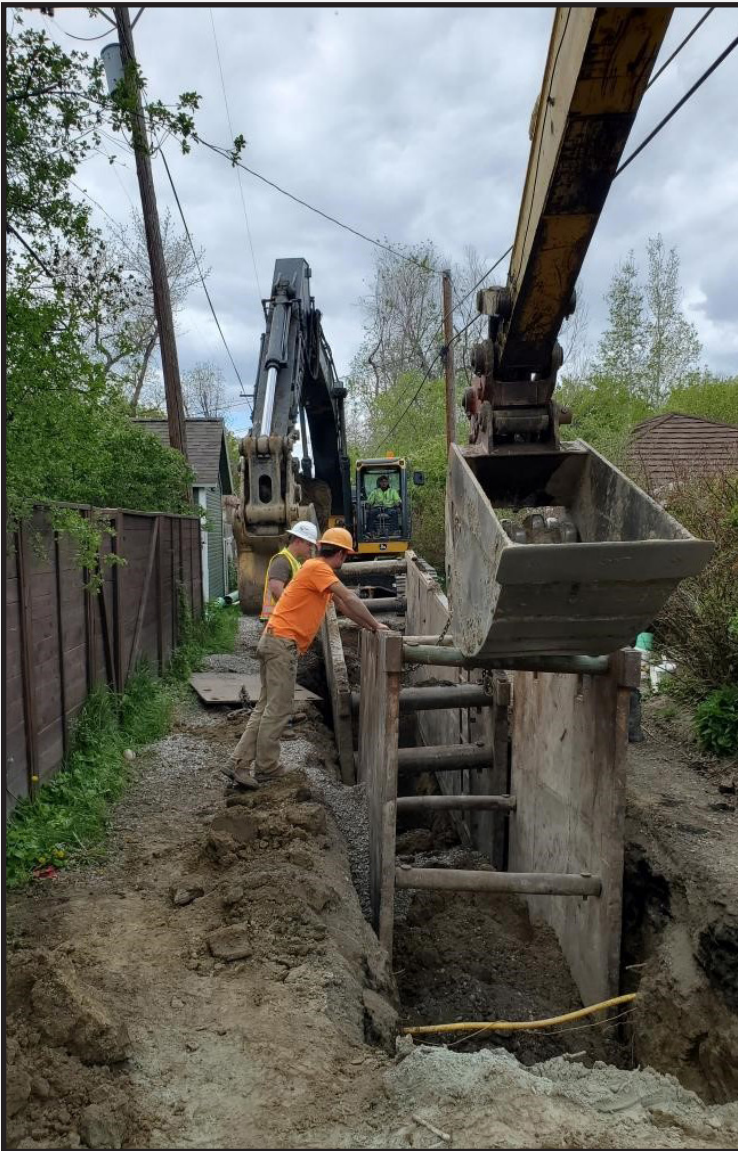
Low overhead utilities.
