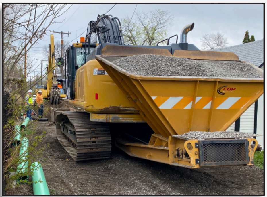
Working in tight conditions. Shown is a bedding conveyor on the lead excavator.
