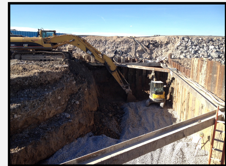
Excavating out the wet well, Komatsu 490 up top and PC 35 in the bottom.
