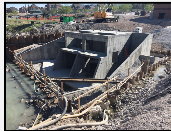
Complete intake structure, waiting to install misc. metals on the structure before pulling sheet pile.
